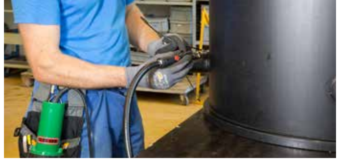
LABOR S, used in combination with MINOR as an external air supply.
