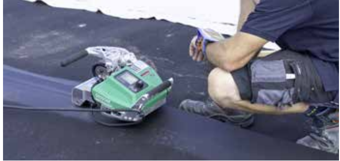
GEOSTAR LQS in field operation.
