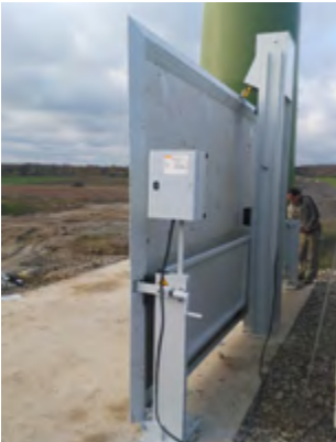
Box for protecting the control
